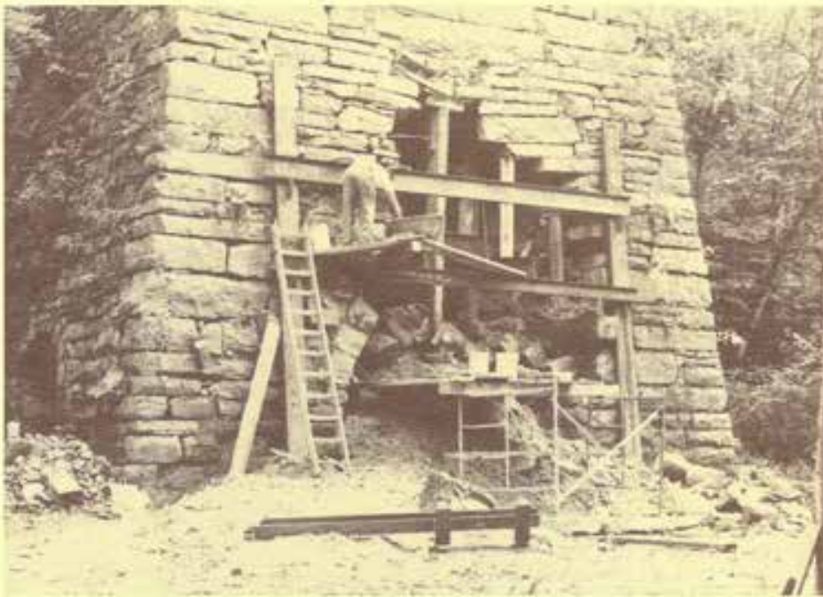
Repair of the casting arch proceeds at Forest Dale State Historic Site (Vic Rolando photo).
